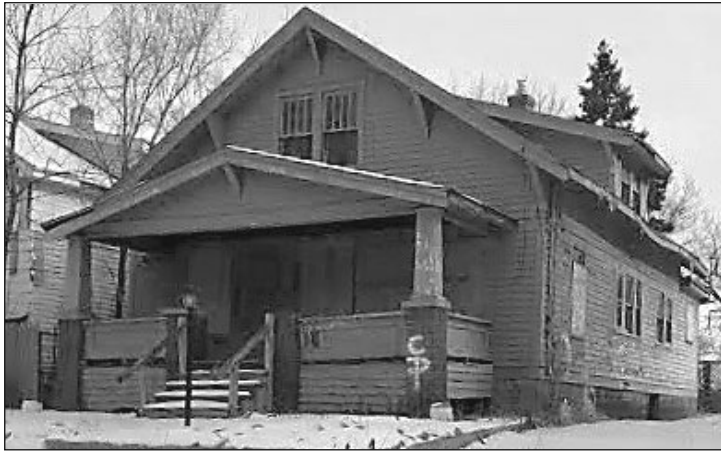
Mabbitt's childhood home on Bennett Avenue, boarded up. (Photo by Melodee Mabbitt)
