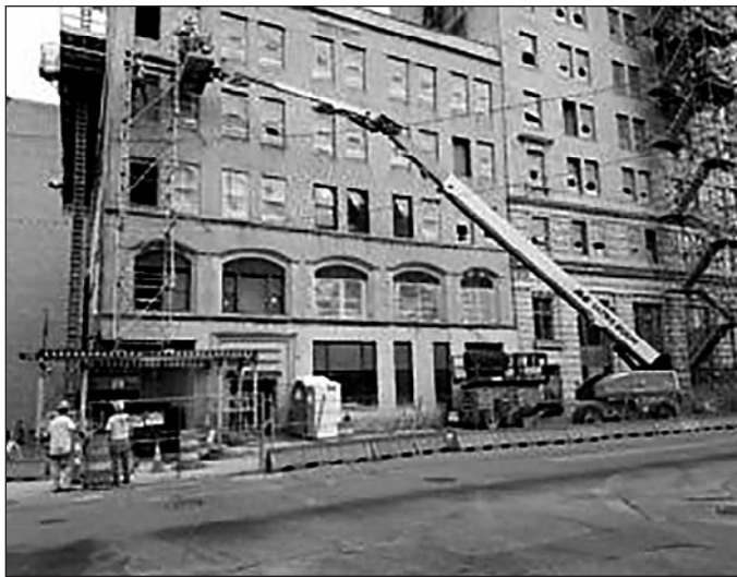
Construction machinery, debris in dumpsters, and street blockages occurred for several months on Kearsley Street during the two year renovation. This photo is from Spring 2020. (Photo by Tom Travis)
