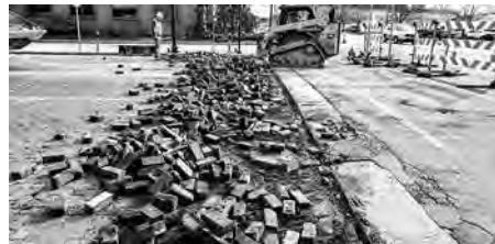
Workers begin tearing out the old bricks at the intersection of Court and Saginaw Streets in April 2023
